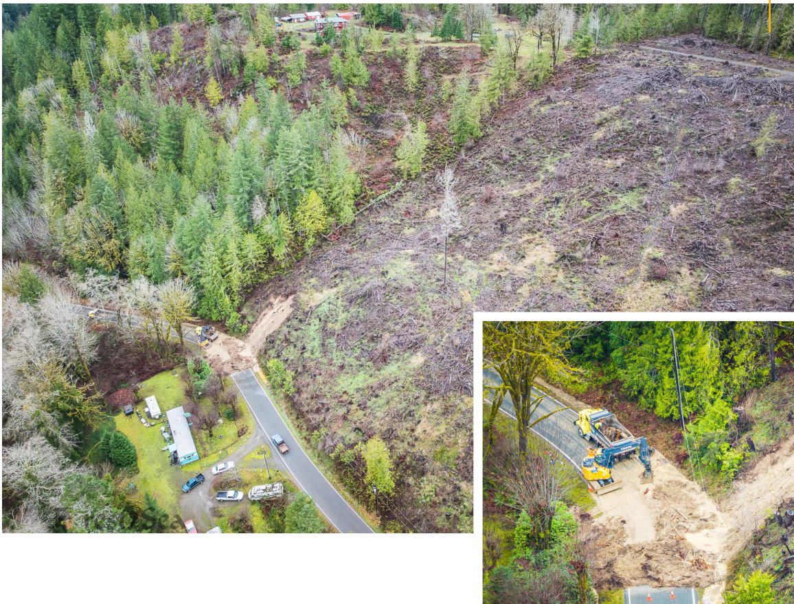
Figure 6. Aldwell Landslide Adjacent to Harvested Area
